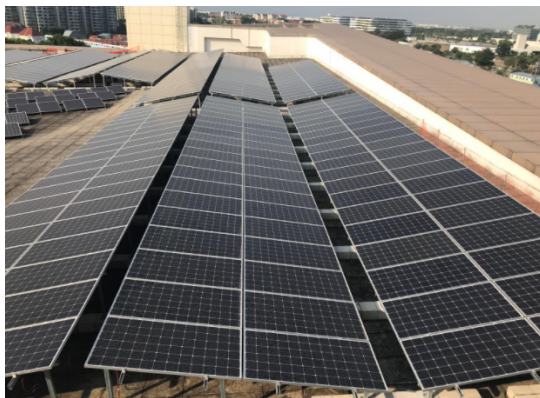
Solar panels at ITE College East. (Photo: ITE)
